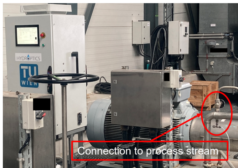
Figure 1: Hydroptics Oil in water module connected to the process stream of OMV WTP
