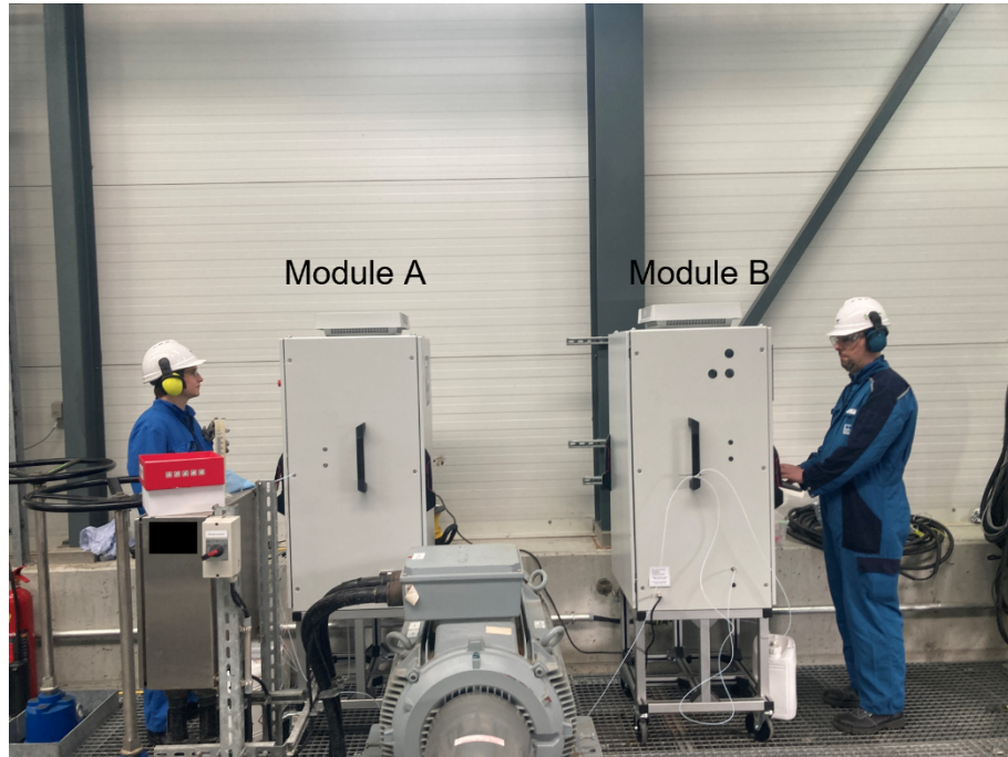
Figure 2: Modules A & B connected and measuring OMV WTP process stream
